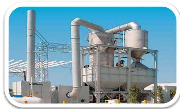
Scrubbers, Vents & Utility Systems
