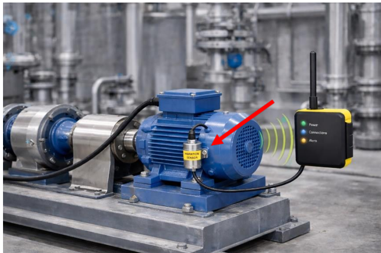
Figure 1. Motor with vibration sensor installed.
