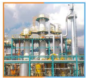
Sulfuric Acid Plant, Turkey
