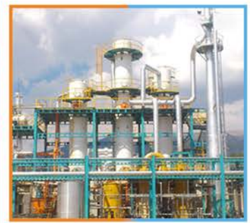
Sulfuric Acid Plant, Turkey
