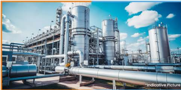
2200 TPD Chlor - Alkali Plant, India
